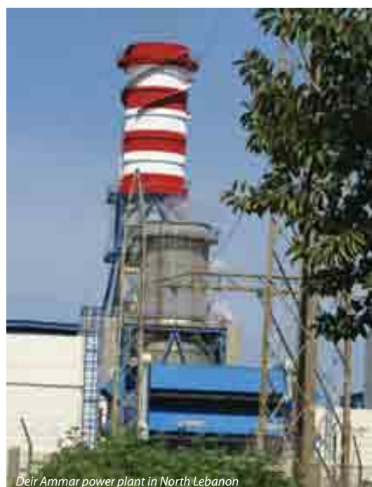
Deir Ammar power plant in North Lebanon
